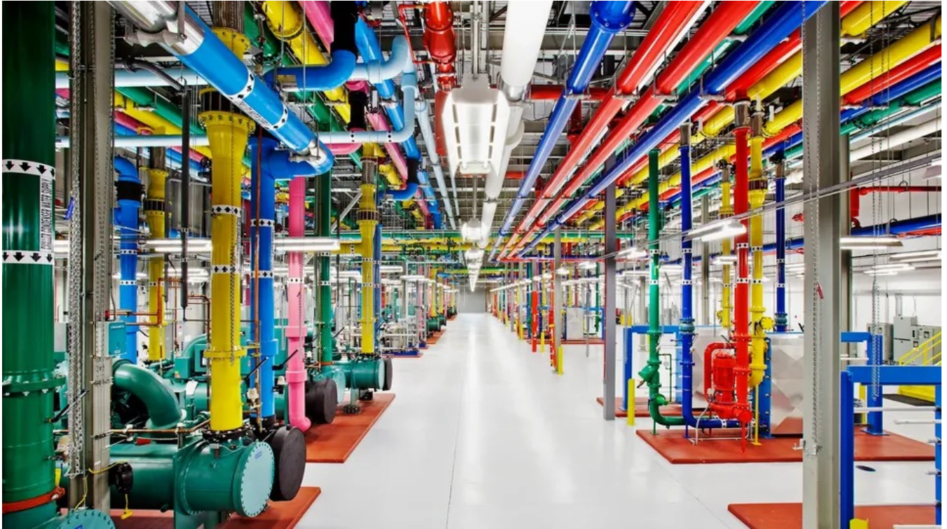
Google-Rechenzentrum in Douglas County, Georgia, USA. Foto: Connie Zhou/AP
